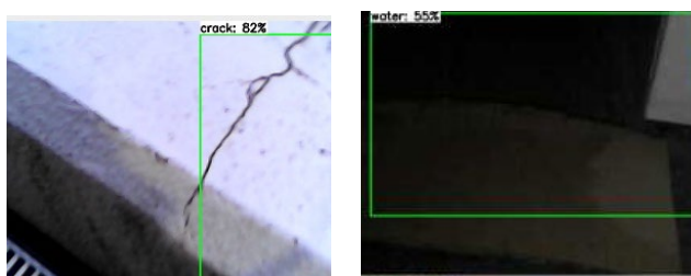
(a) Crack recognition by the robot (b) Water recognition by the robot Fig. 9. Object detection result.
